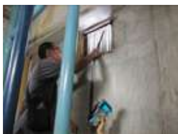
Sample Measurement in AHU Room
